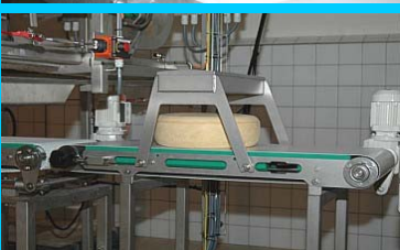
TS-rating at conveyor-belt
